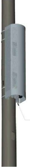
Figure 1 - Example of an antenna enclosure with a curved shape side-mounted to a pole
