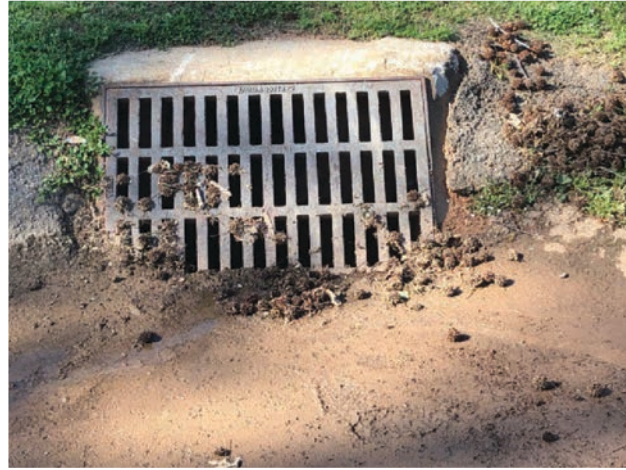
(example of one of the drainage grates at the park)
